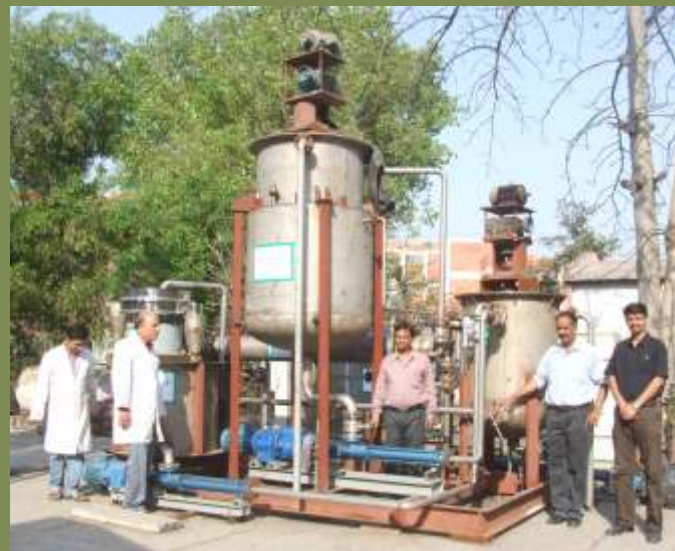
Commissioning of Pilot Plant for Removal of Non Process Elements at CPPRI
